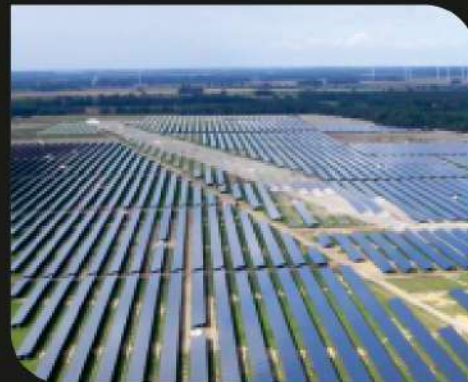
Dholera 5000 MW TATA Solar Plant
